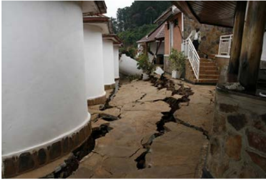
Fig.1. Surface faultings, landslides and significant damage to human infrastructures.
